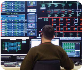
Command and Control Rooms
