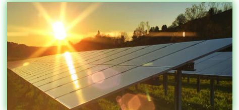
Power and Energy Management
